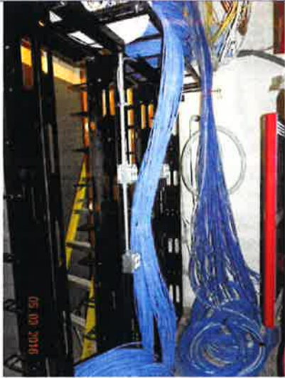
1st Floor IT Room
