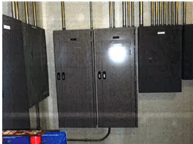
1st Floor Electrical Room
