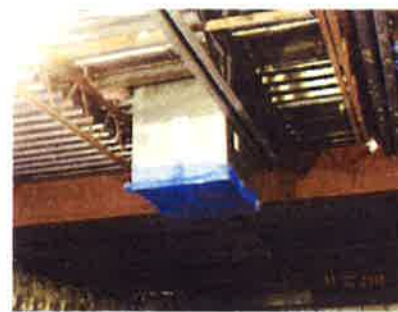
Ductwork from Rooftop Unit
