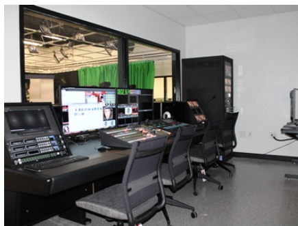
Studio Control Room
