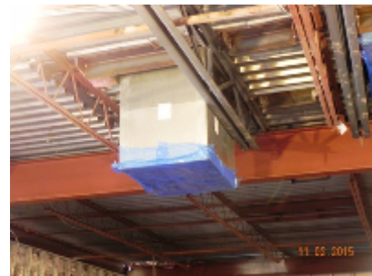
Ductwork from Rooftop Unit
