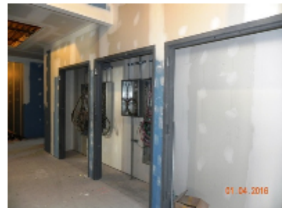
2nd Floor Electrical Panels
