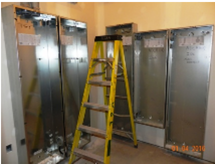
1st Floor Electrical Panels
