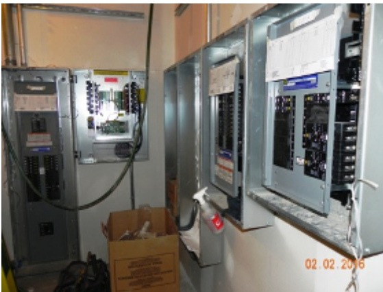
1st Floor Electrical Panels
