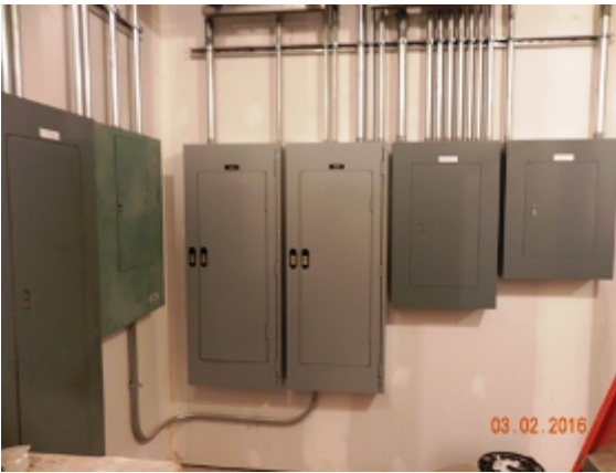
1st Floor Electrical Panels
