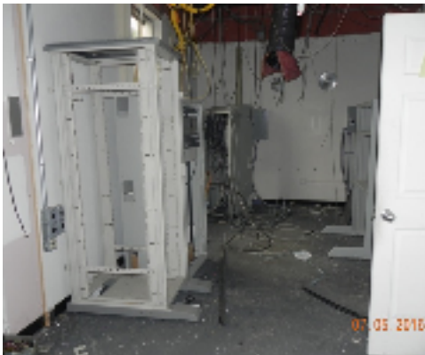
2nd Floor IT Server Room
