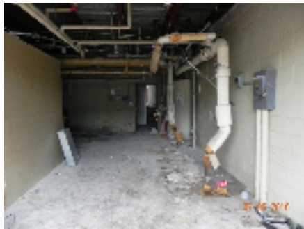
Old D.O. Mechanical Room
